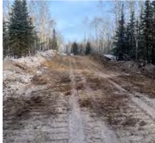
Finished Product of dozer at KP 143.3, Mulch on left and side slope material on right.
